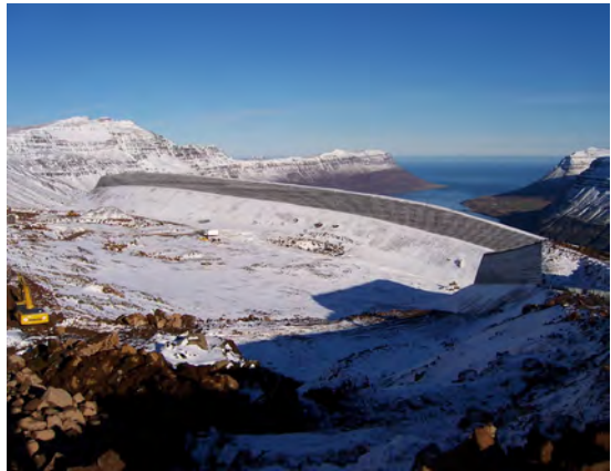
Reinforced Earth® avalanche barrier, Seydisfjurdur (Islande)
