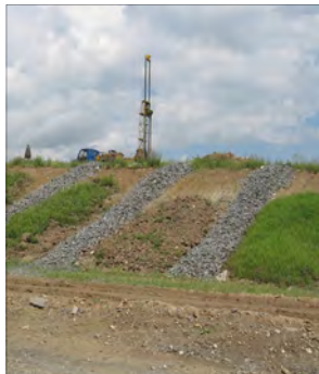
Fig. 1: Drilling works in the slope deformation location and defects caused by diatomaceous earth.
